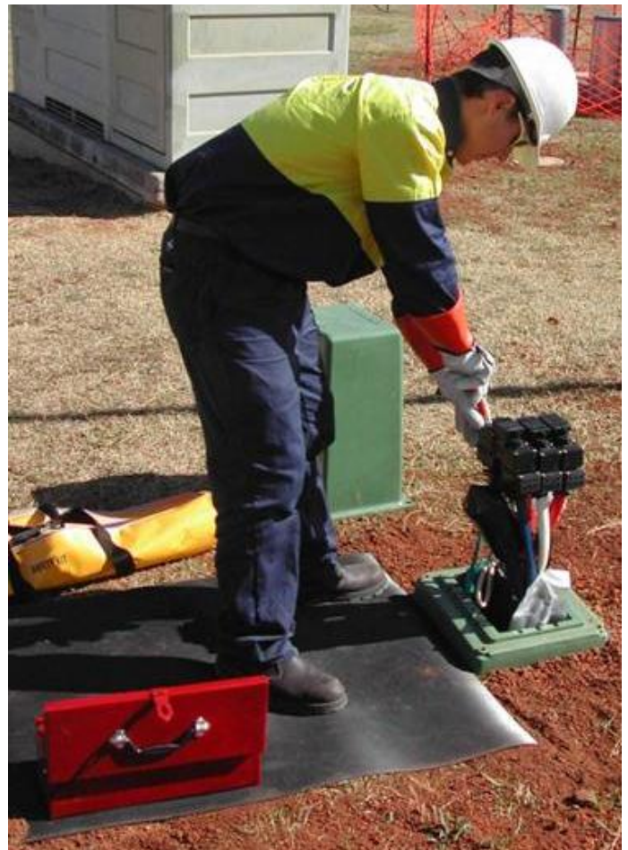
Figure 1. Live Low Voltage work practices being applied during work on underground distribution mains at a pillar
